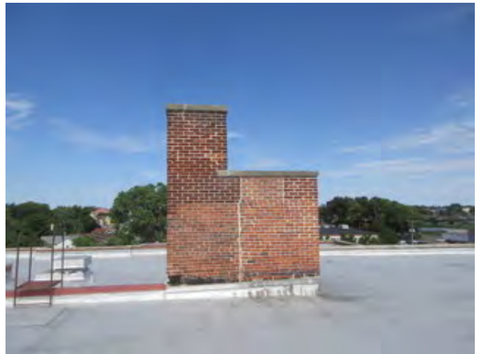
Chimney Tuckpointing Required
