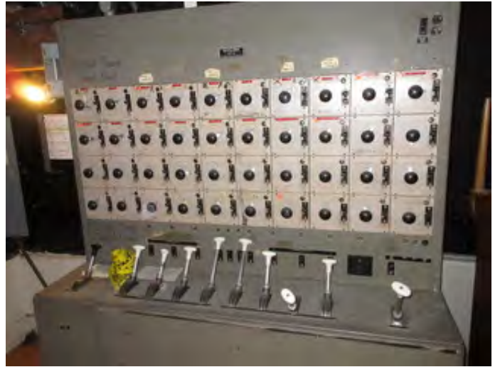
Stage Control Panel
