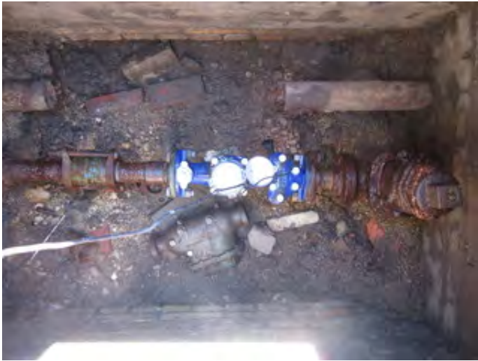
Incoming Domestic Water Service Line
