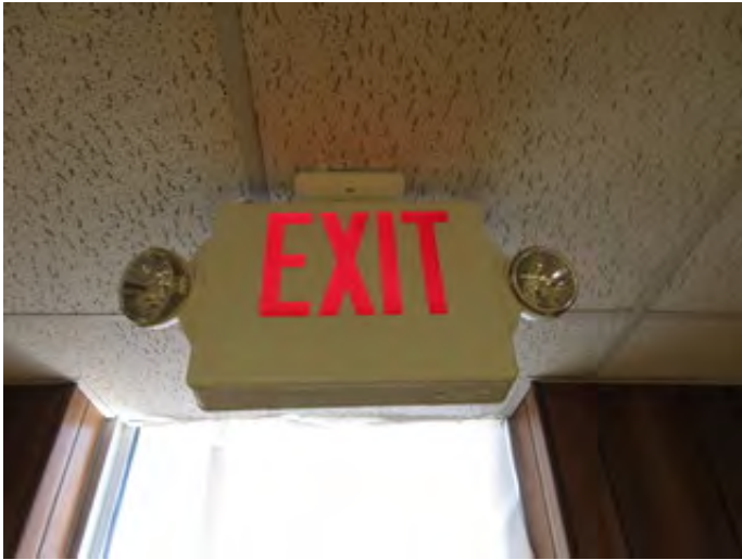
Exit Sign with Emergency Egress Lighting
