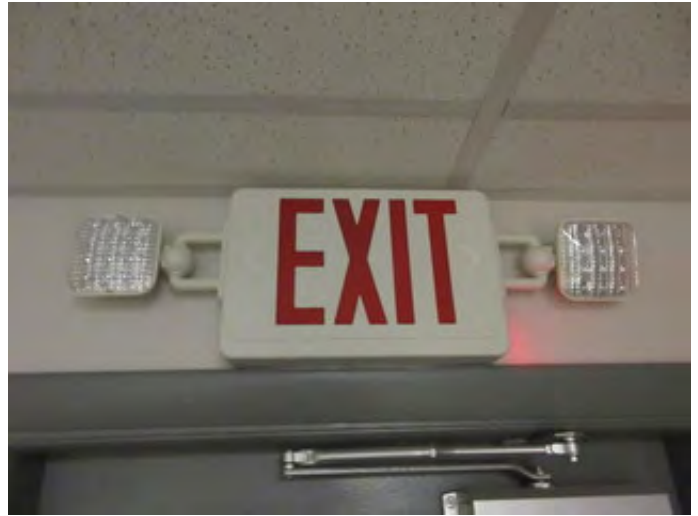
Exit Sign with Emergency Egress Lighting
