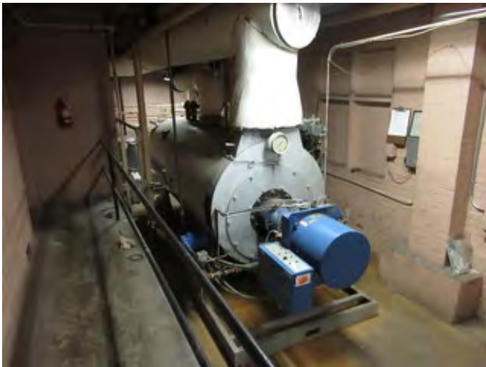
Natural Gas Fired Boiler
