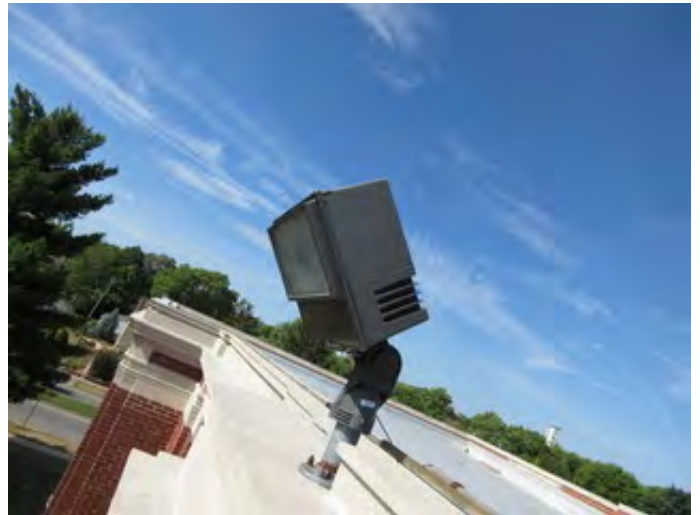
Exterior Entry Light Fixture
