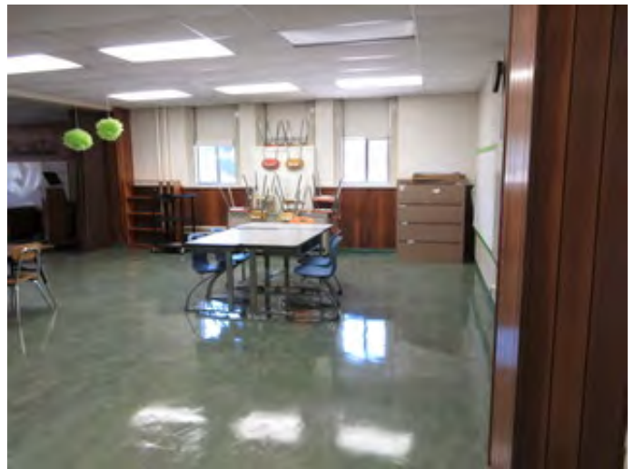
Classroom Fluorescent Lighting Fixtures
