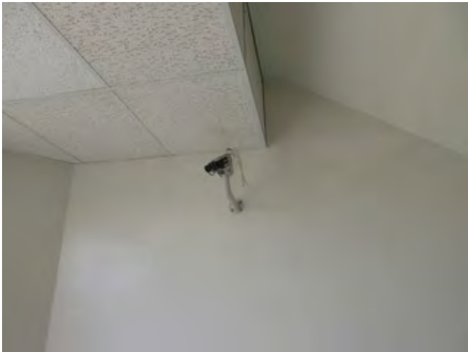
Security System CCTV Camera
