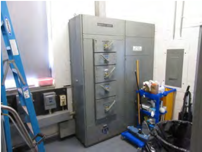
Main Electrical Distribution Panel
