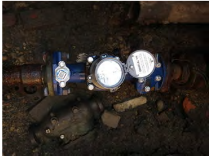
Incoming Domestic Water Service Meter
