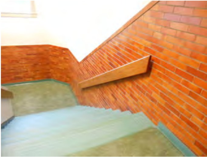
Non Compliant Stair Tower
