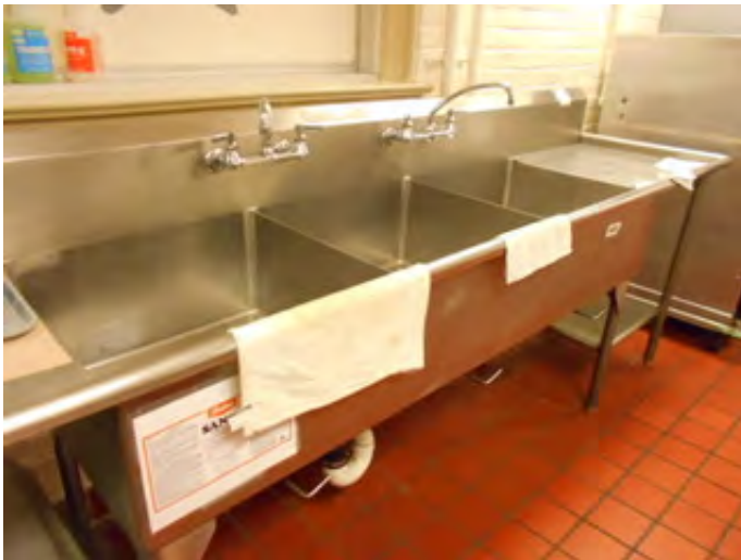
Triple Compartment Sink-Kitchen
