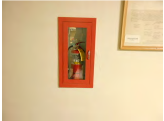
Compliant Fire Extinguisher
