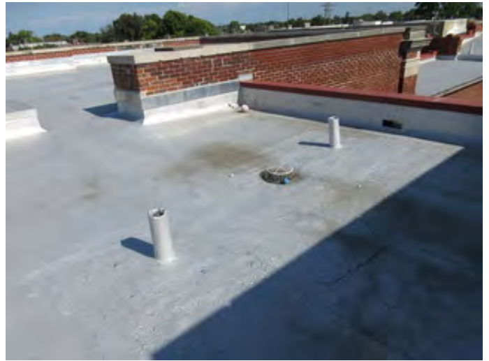
Waste Vent Piping
