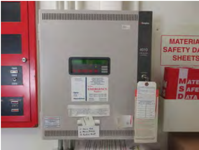
Fire Alarm System Control Panel
