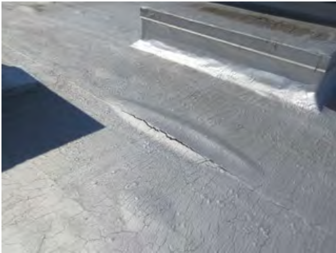
Typical Blisters & Cracking
