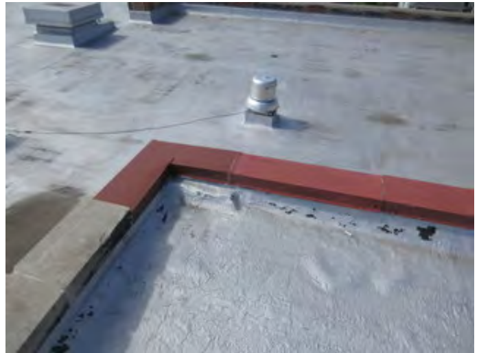
Blisters and Metal Coping
