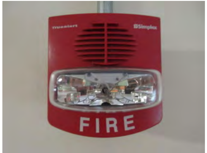
Fire Alarm System Audible Horn and Visual Strobe Device
