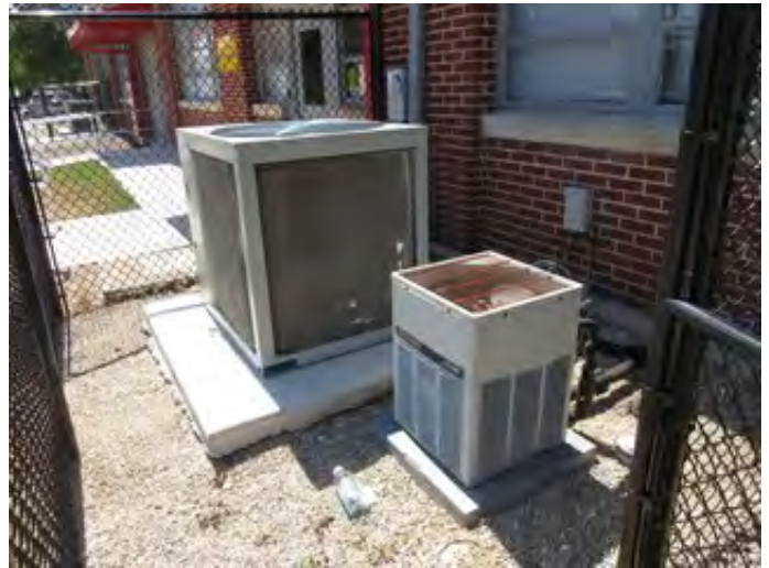
Air Condition System Condenser
