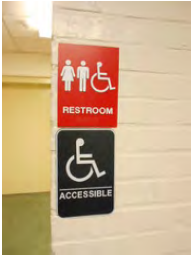
ADA Compliant Signage-Interior
