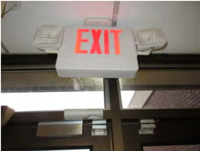
Exit Sign with Emergency Egress Lighting
