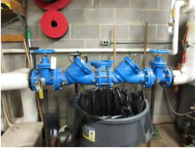
Incoming Domestic Water Service Line
