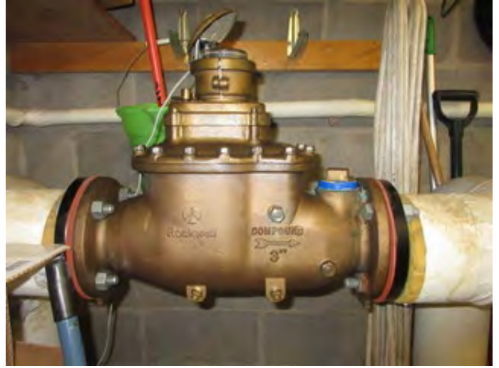
Incoming Domestic Water Service Meter
