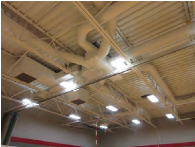
Gymnasium Fluorescent Lighting Fixtures
