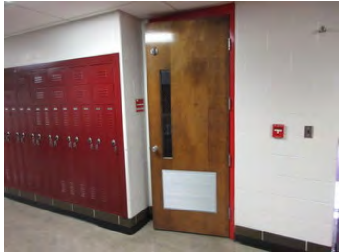
Fire Alarm System Manual Pull Station
