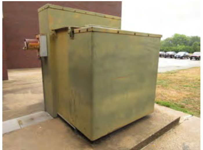
Pad Mounted Transformer
