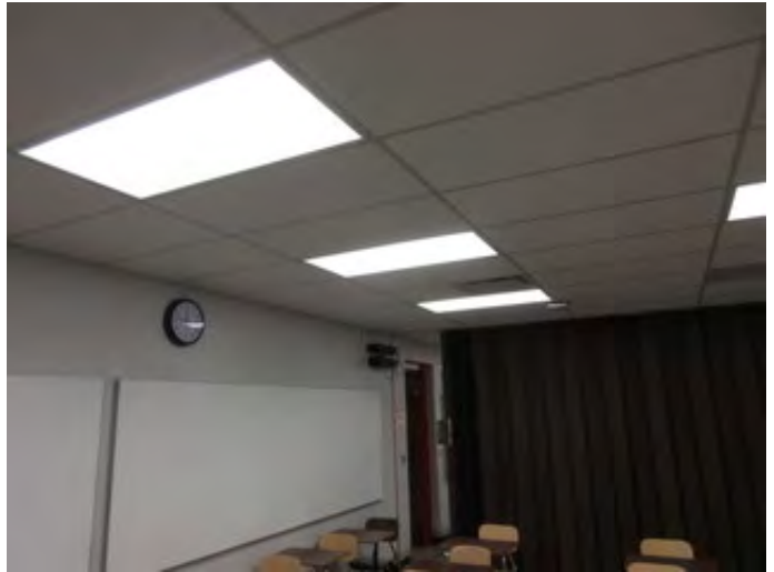
Classroom Fluorescent Lighting Fixtures
