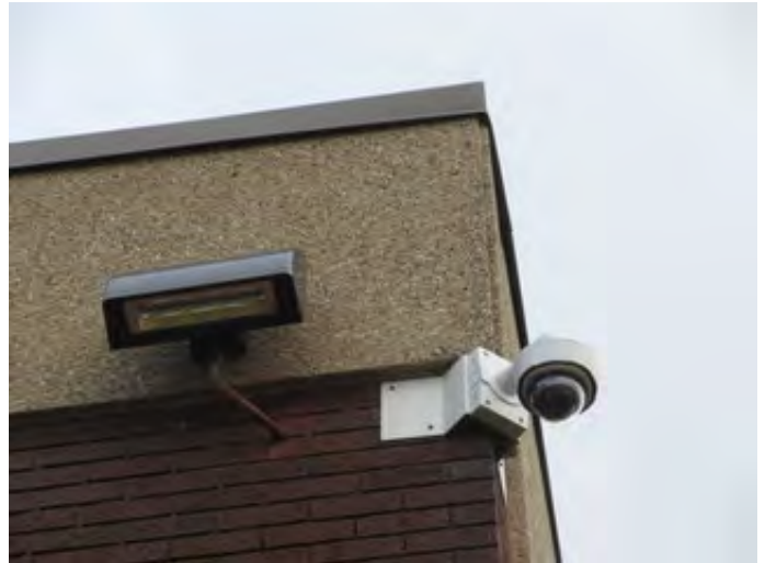
Security System CCTV Camera
