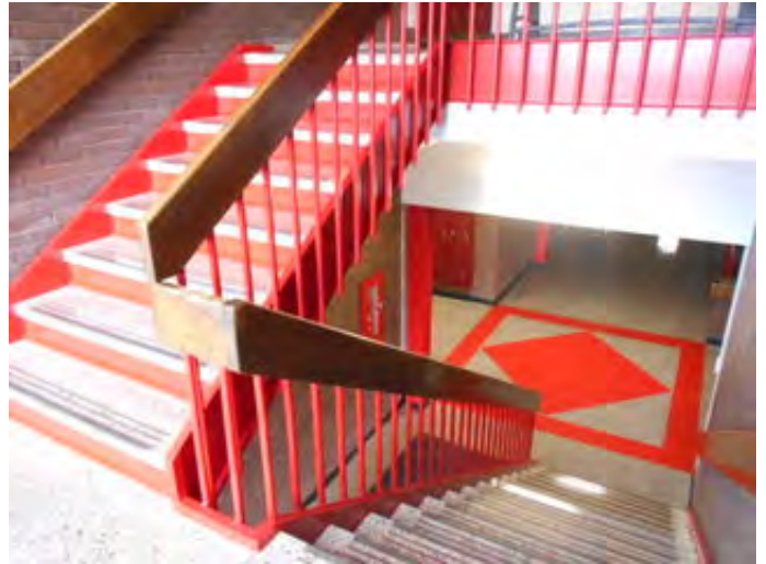
Non-Compliant Stair Tower
