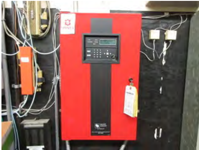
Fire Alarm System Control Panel
