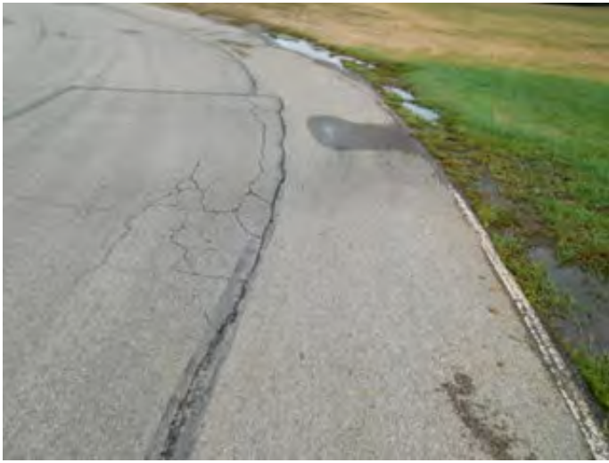
Ponding at Pavement Edges
