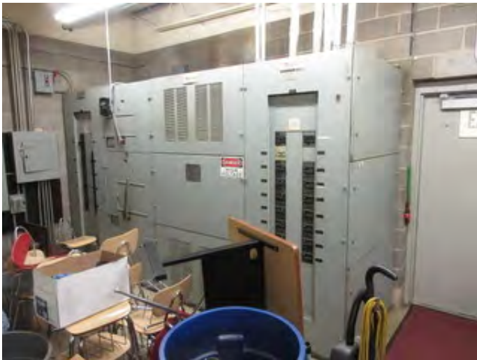
Main Electrical Distribution Panel
