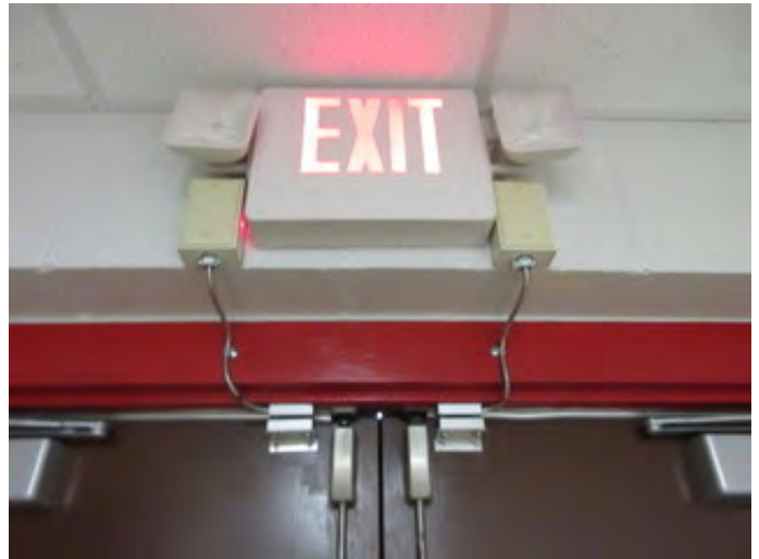
Exit Sign with Emergency Egress Lighting
