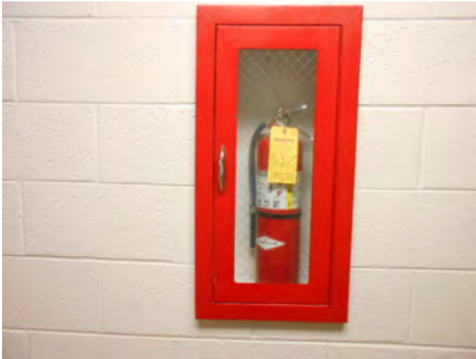
Compliant Fire Extinguisher
