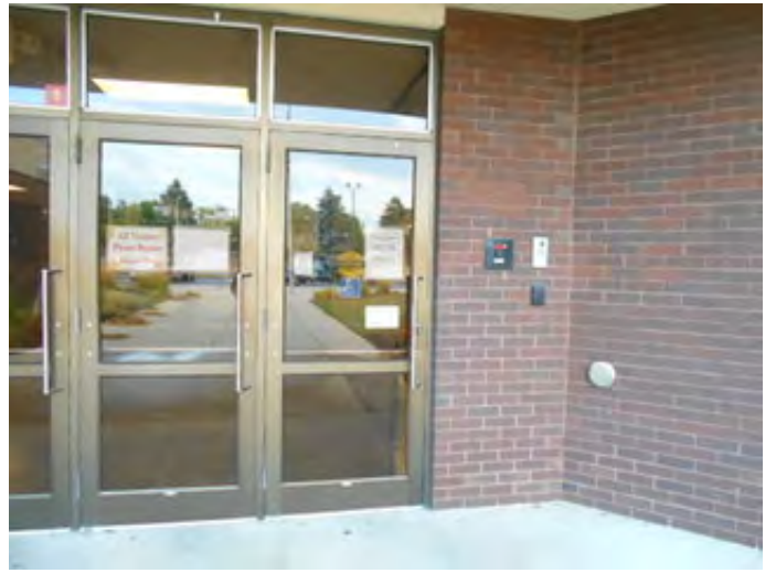
Compliant Power Assisted Door
