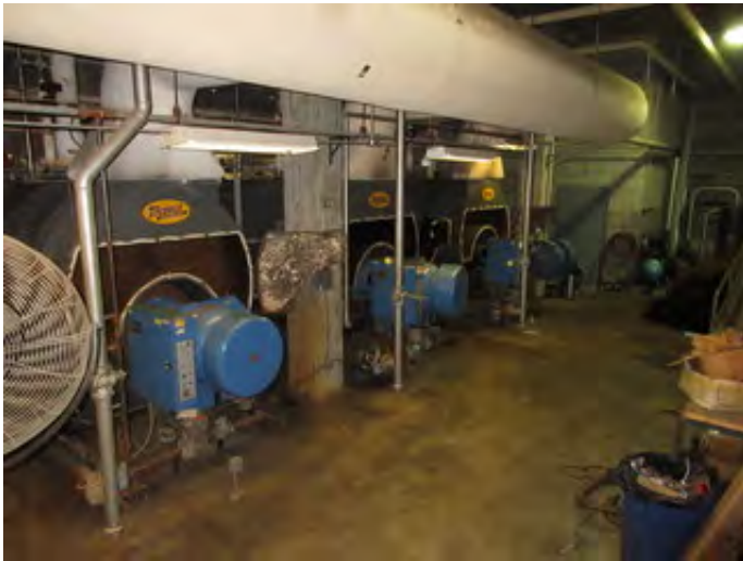
Natural Gas Fired Heated Water Boilers
