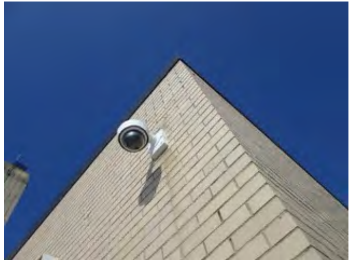
Security System CCTV Camera
