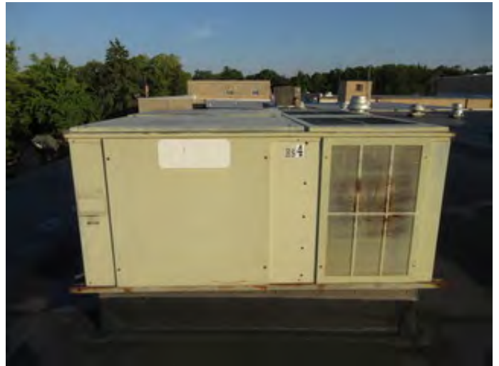
Packaged Roof Top Unit
