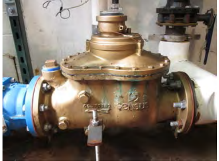
Incoming Domestic Water Service Meter
