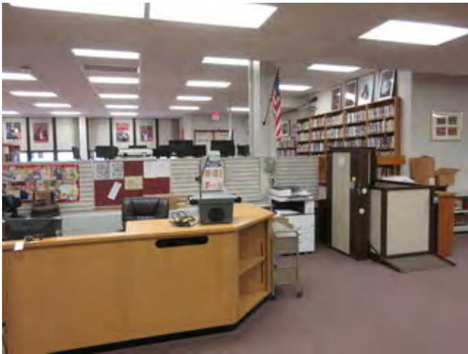
Media Center Fluorescent Light Fixtures
