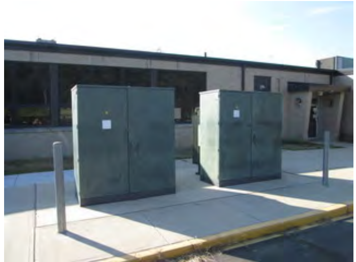
Pad Mounted Transformers
