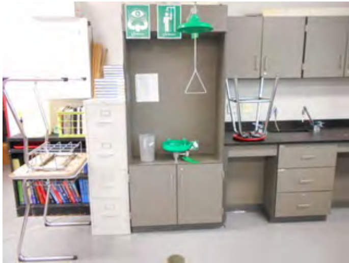
Emergency Shower and Eyewash-2006 Addition
