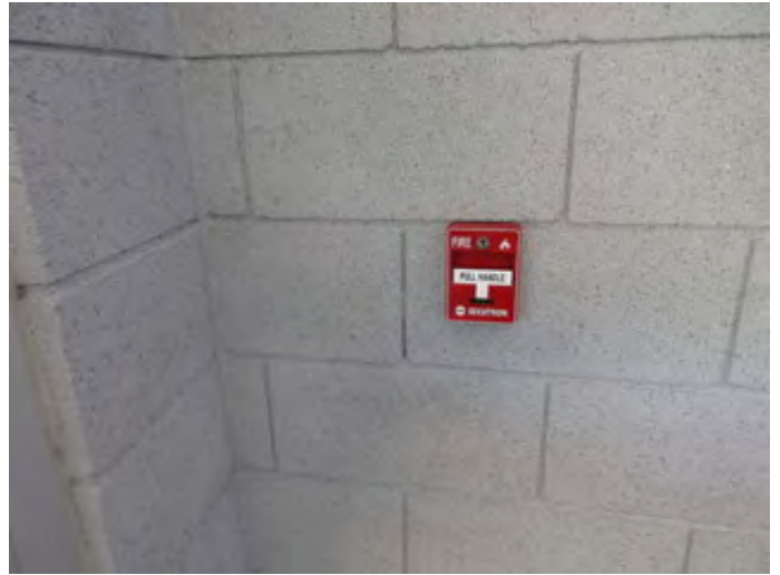
Fire Alarm System Manual Pull Station
