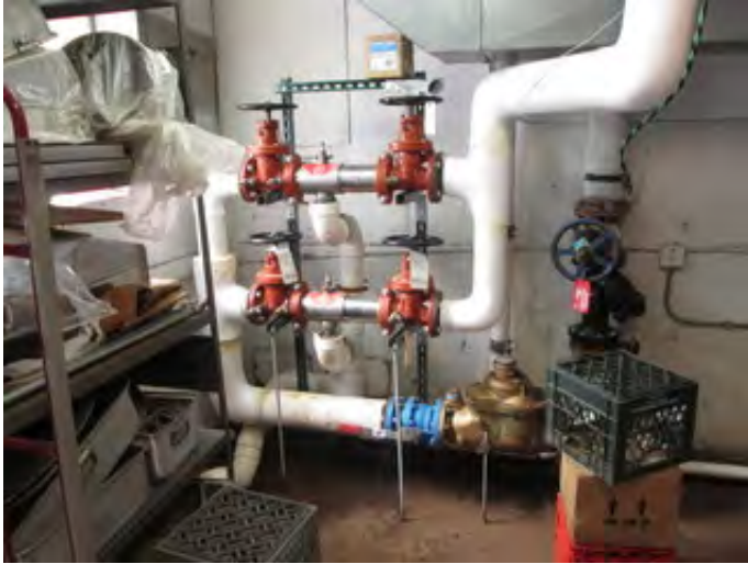
Incoming Domestic Water Service Line
