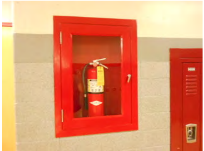
Compliant Fire Extinguisher
