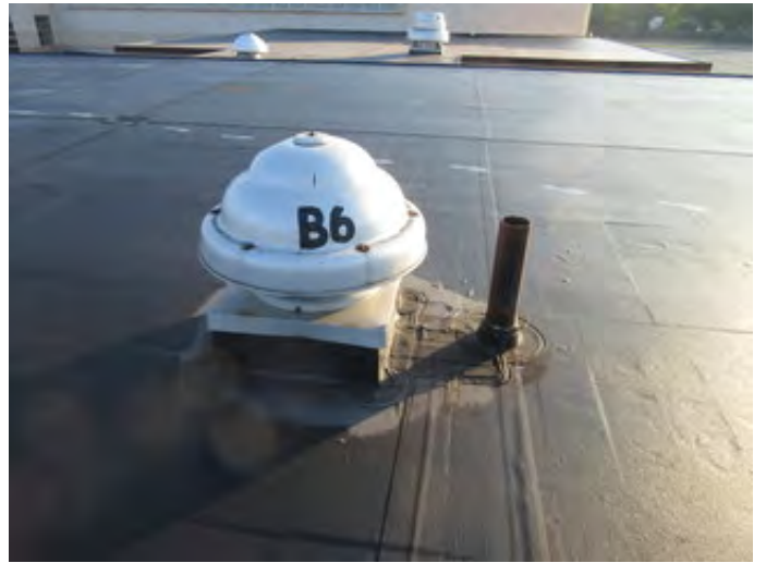
Waste Vent Piping
