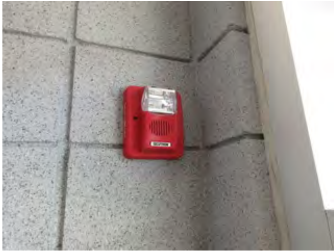
Fire Alarm System Audible Horn and Visual Strobe Indicating Device
