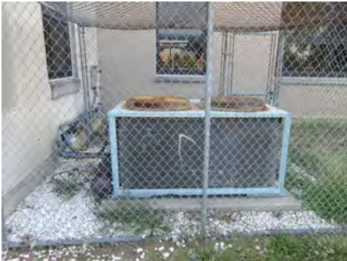
Ducted Split HVAC Condensing Units
