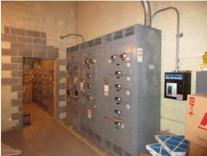
Main Electrical Distribution Panel
