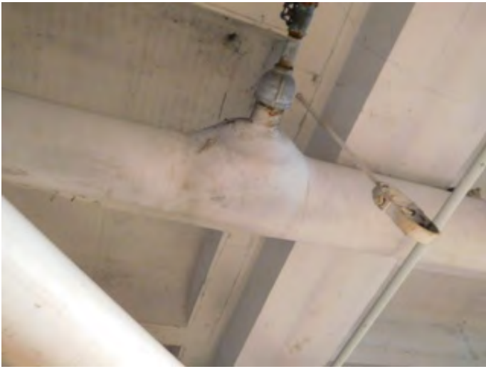
Mud Pipe Insulation
