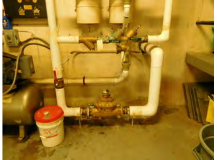
Incoming Domestic Water Service Line
