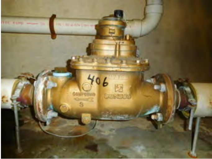
Incoming Domestic Water Service Meter
