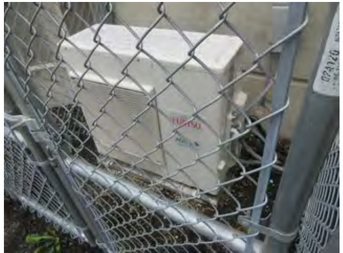
Ductless Split AC Condensing Unit
