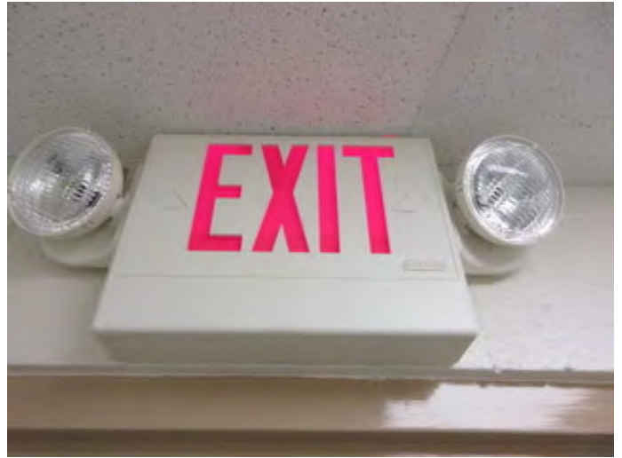
Exit Sign with Emergency Egress Lighting
