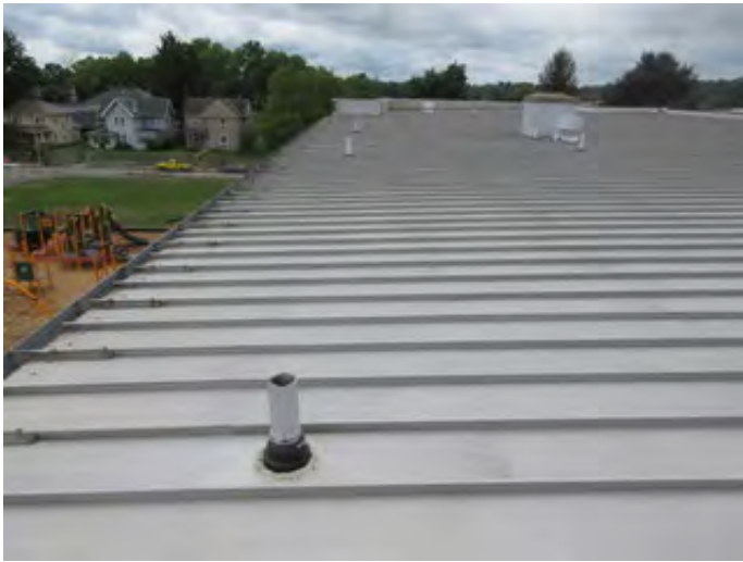
Waste Vent Piping
