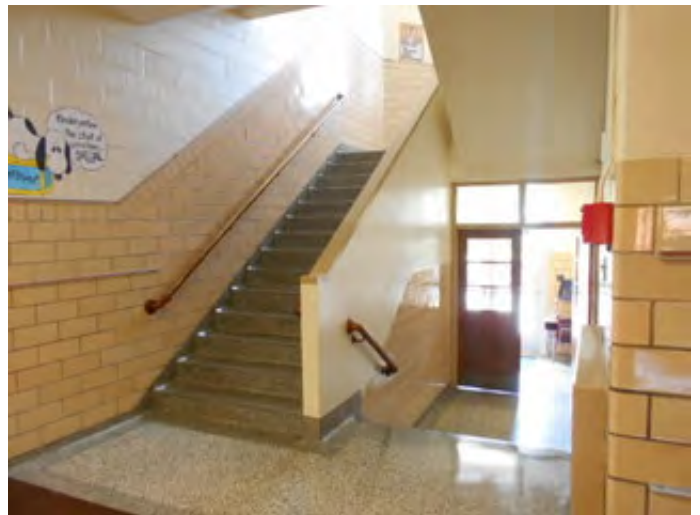
Non-Compliant Stair Tower
