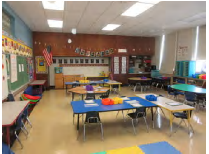
Classroom Fluorescent Light Fixtures
