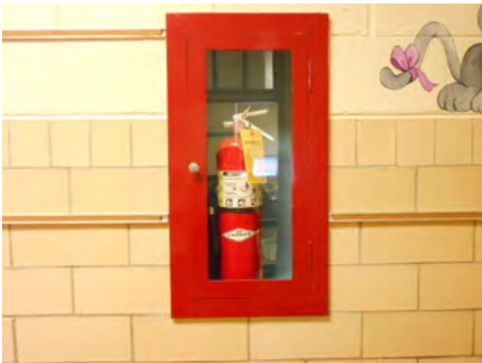
Compliant Fire Extinguisher
