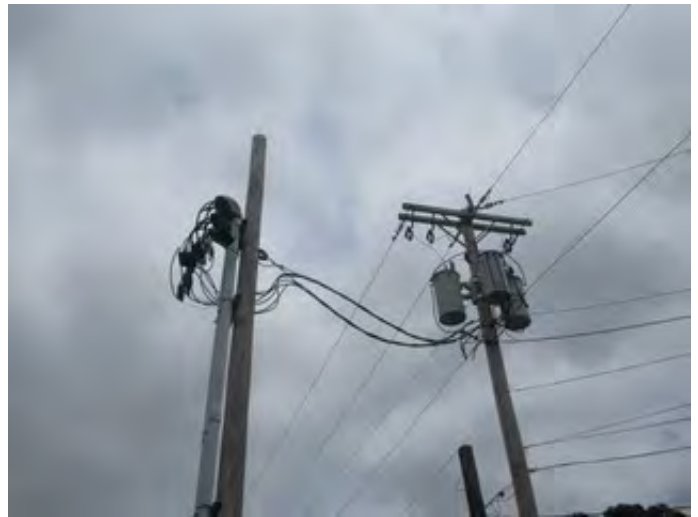
Pole Mounted Transformers
