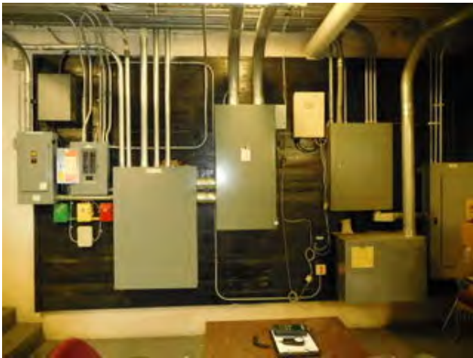
Main Electrical Distribution Panels
