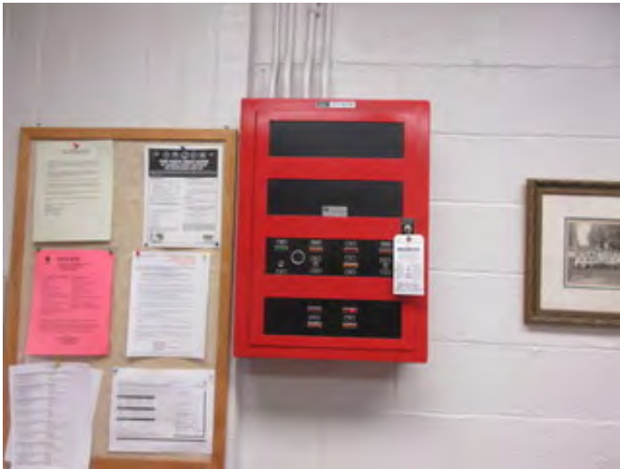
Fire Alarm System Control Panel
