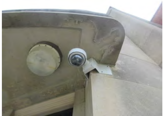
Security System CCTV Camera
