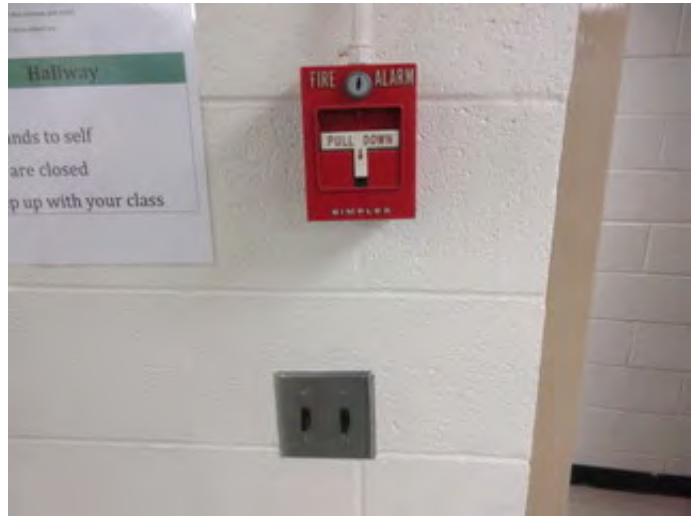
Fire Alarm System Manual Pull Station
