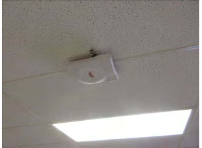
IT Wireless Access Point
