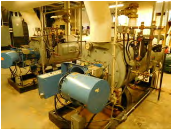
Natural Gas Fired Heated Water Boilers
