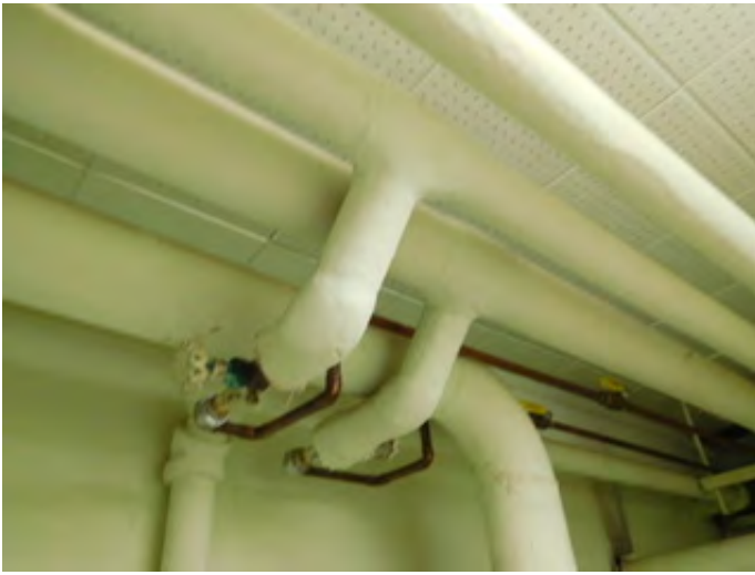
Mud Elbow Fittings and Pipe Insulation
