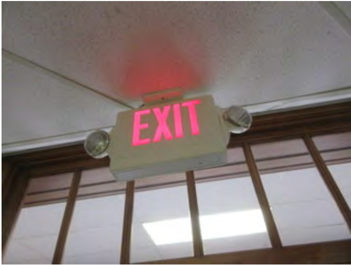
Exit Sign with Emergency Egress Lighting
