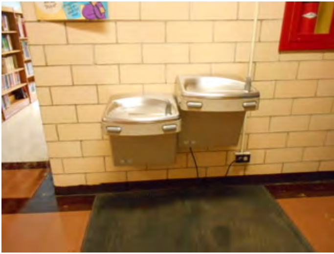
Electric Water Coolers
