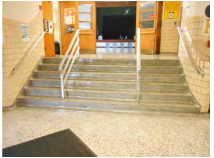
Non-Compliant Access to Gym/Cafeteria
