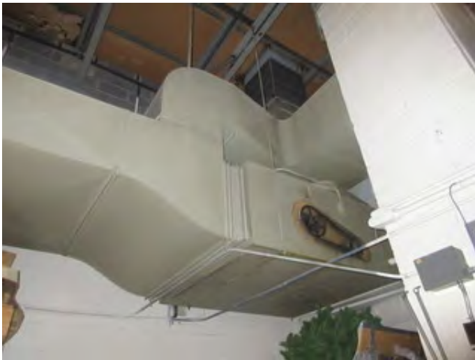
Air Handling Unit
