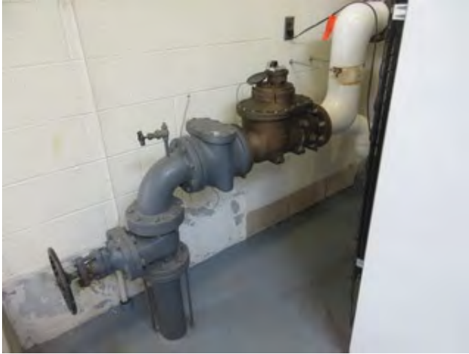
Incoming Domestic Water Service Line
