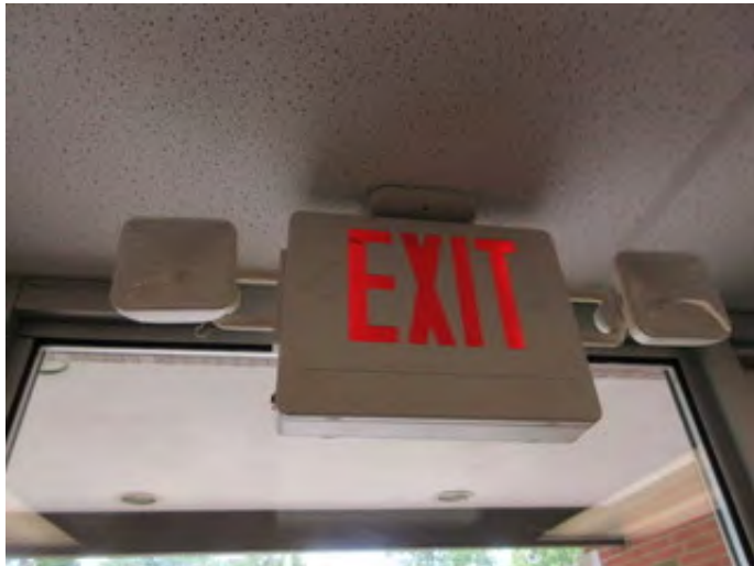
Exit Sign with Emergency Egress Lighting
