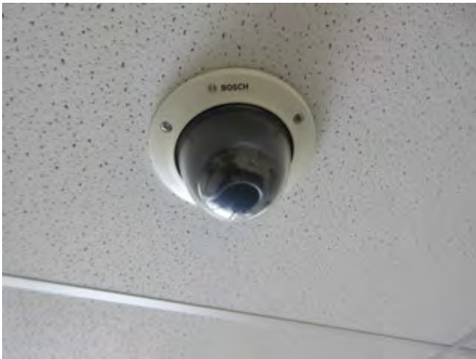
Security System CCTV Camera
