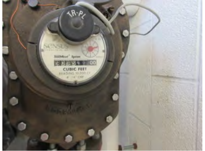
Incoming Domestic Water Service Meter
