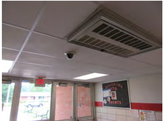
Exit Sign with Emergency Egress Lighting
