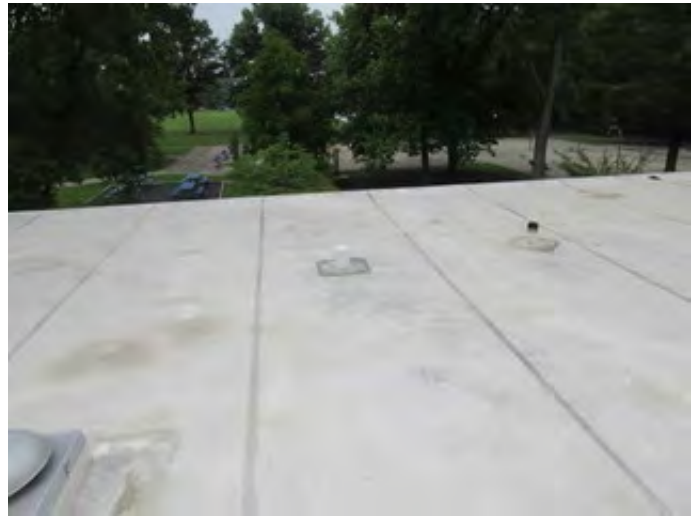
Waste Vent Piping
