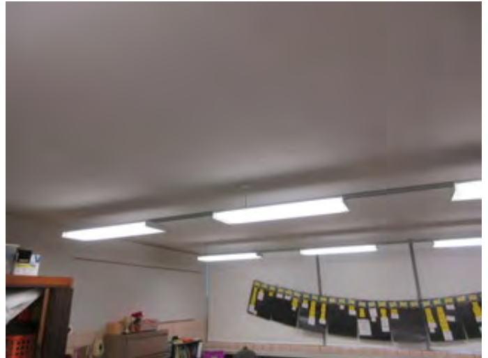
Classroom Fluorescent Light Fixtures
