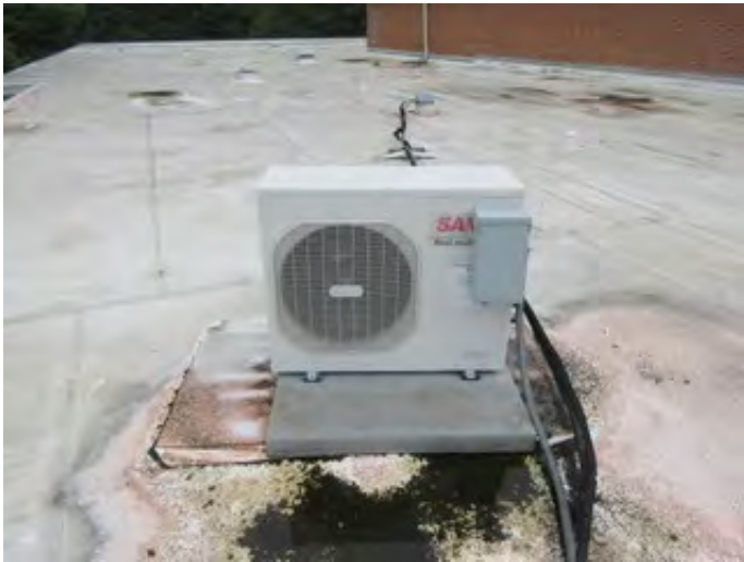
AC Split Condenser
