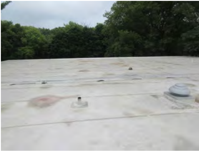
Waste Vent Piping
