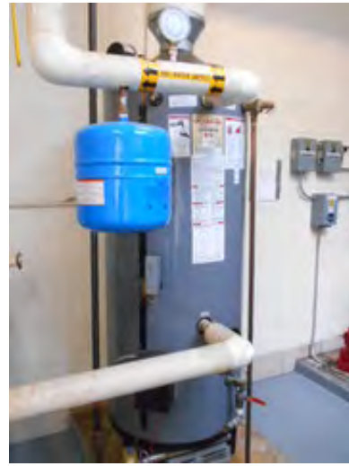
91 Gallon Gas Water Heater
