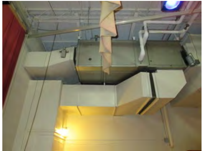
Air Handling Unit
