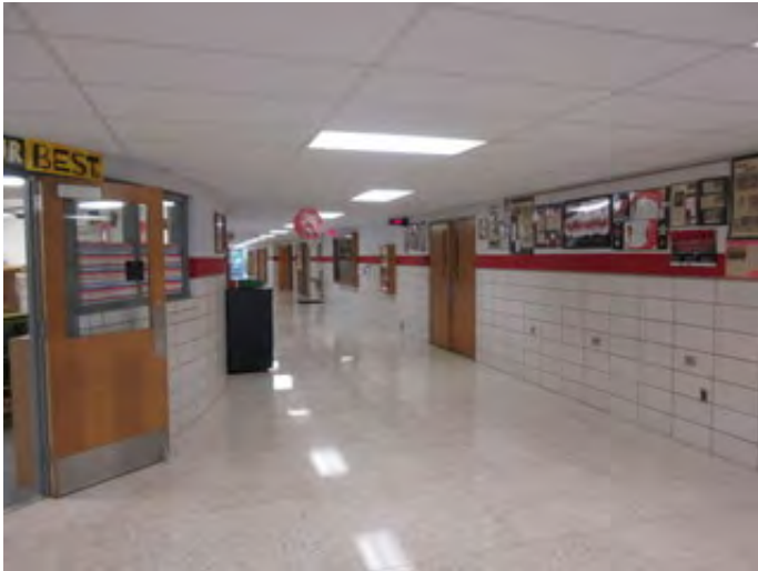
Corridor Fluorescent Light Fixtures
