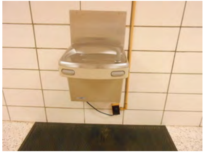
ADA Compliant Electric Water Cooler
