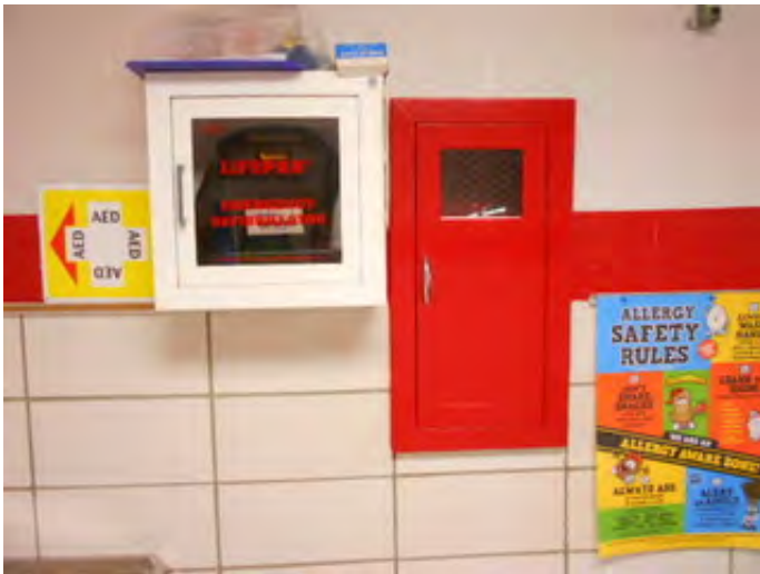
Compliant Fire Extinguisher
