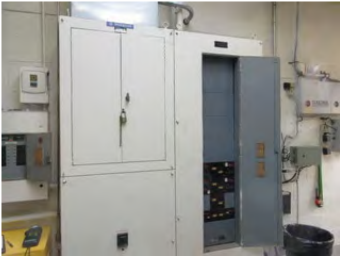
Main Electrical Distribution Panel
