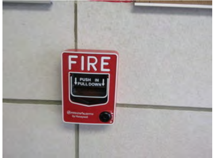
Fire Alarm System Manual Pull Station
