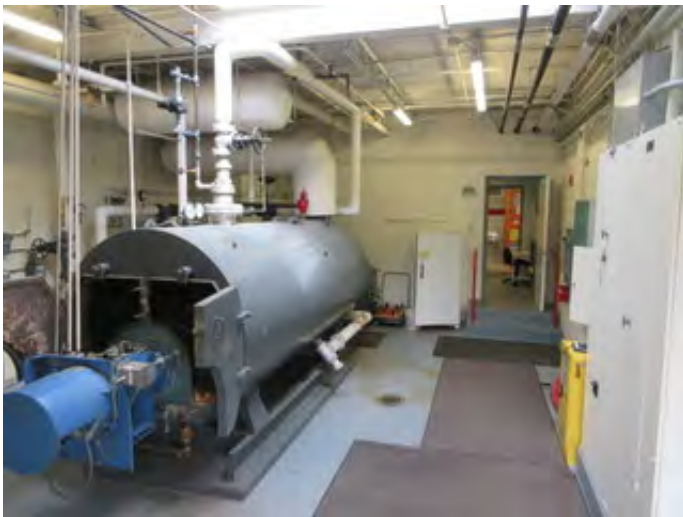
Natural Gas Fired Heated Water Boiler
