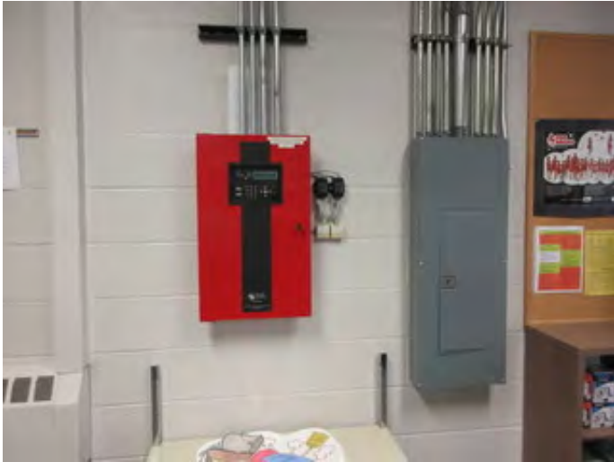
Fire Alarm System Control Panel
