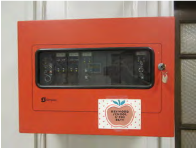
Fire Alarm System Control Panel
