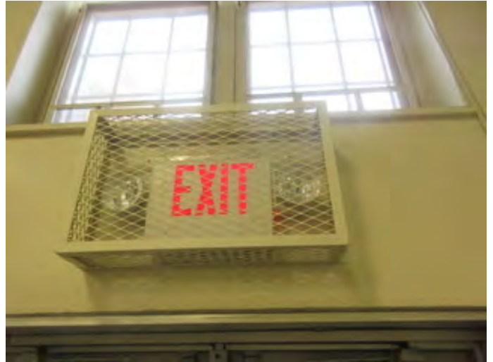
Exit Sign with Emergency Egress Light Fixture
