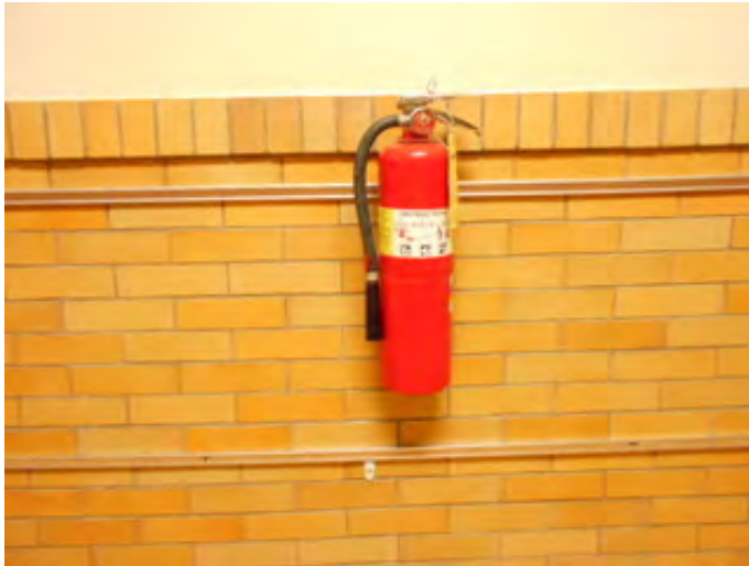
Compliant Fire Extinguisher
