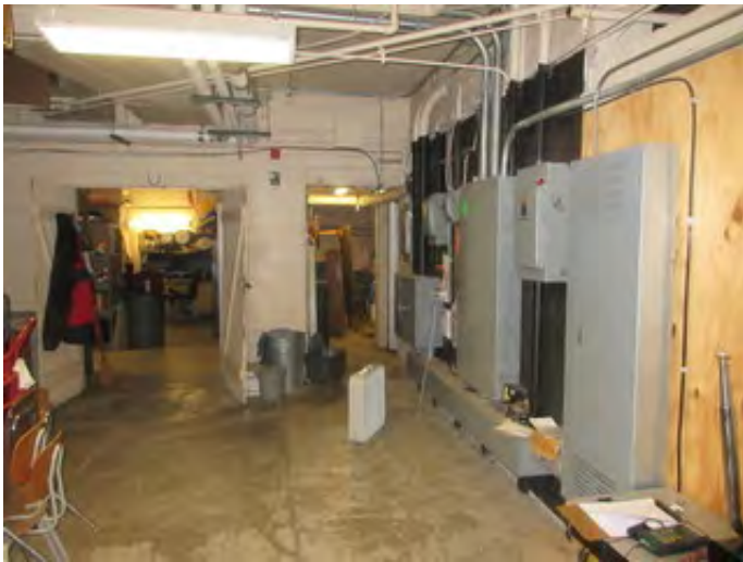
Main Electrical Distribution Panel
