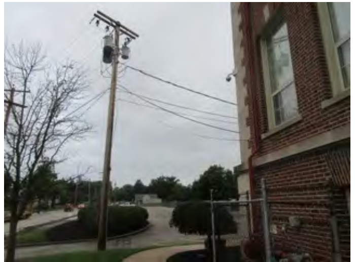
Pole Mounted Transformers
