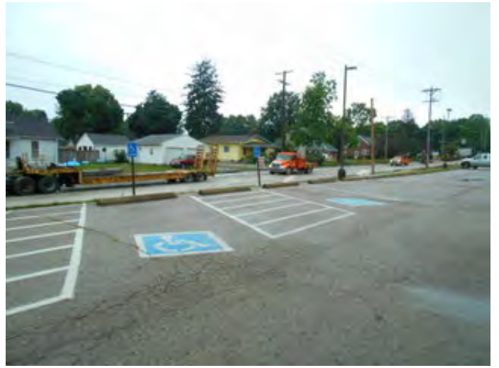
Compliant Handicap Parking
