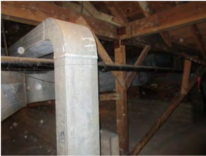
Sanitary Waste Piping
