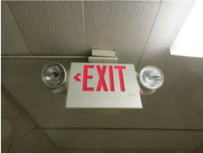
Exit Sign with Emergency Egress Light Fixture
