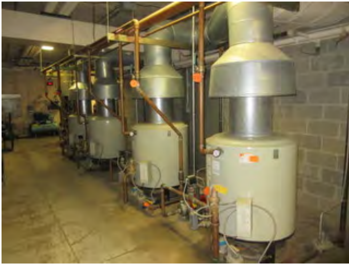
Natural Gas Fired Heated Water Boilers
