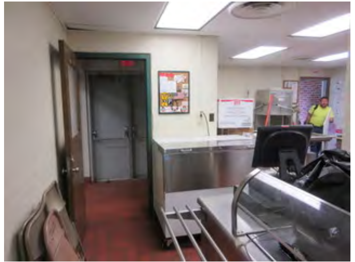
Kitchen Fluorescent Light Fixtures
