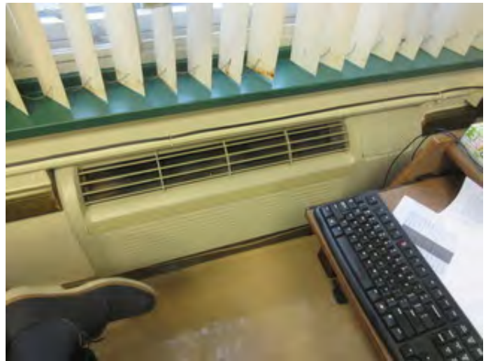
Thru-Wall HVAC Unit
