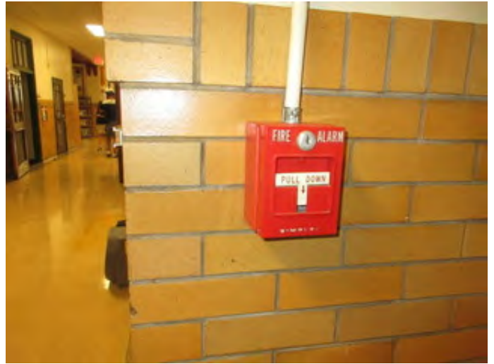
Fire Alarm System Manual Pull Station
