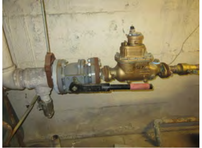
Incoming Domestic Water Meter
