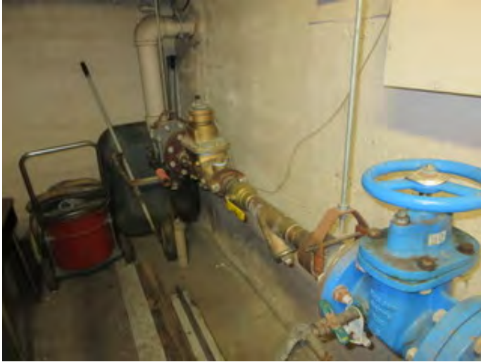
Incoming Domestic Water Service Line
