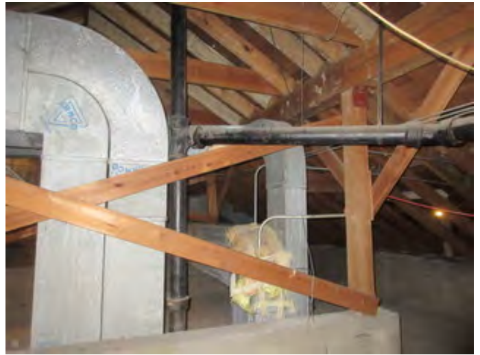
Sanitary Waste Piping
