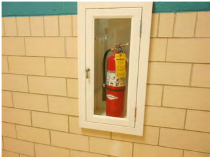
Compliant Fire Extinguisher
