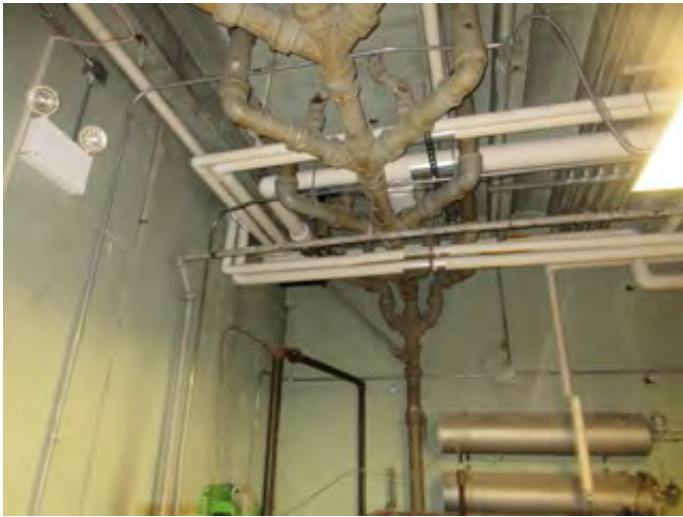
Sanitary Waste Piping
