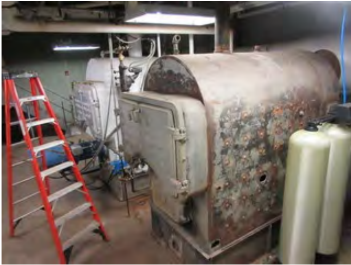
Natural Gas Fired Steam Boilers
