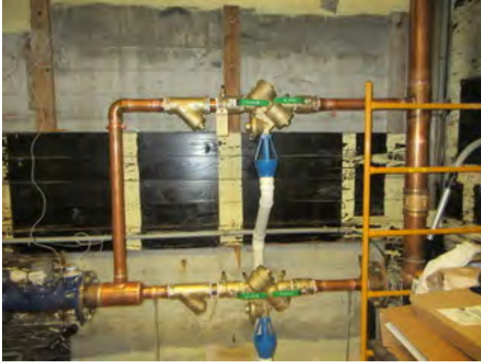
Incoming Domestic Water Service Line
