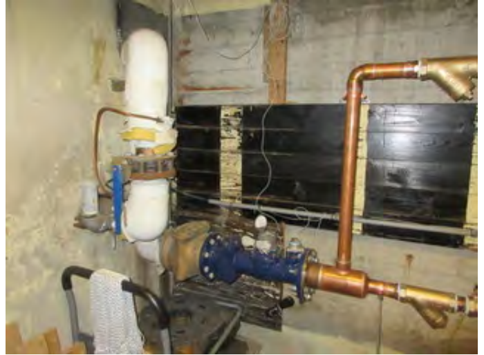
Incoming Domestic Water Service Meter
