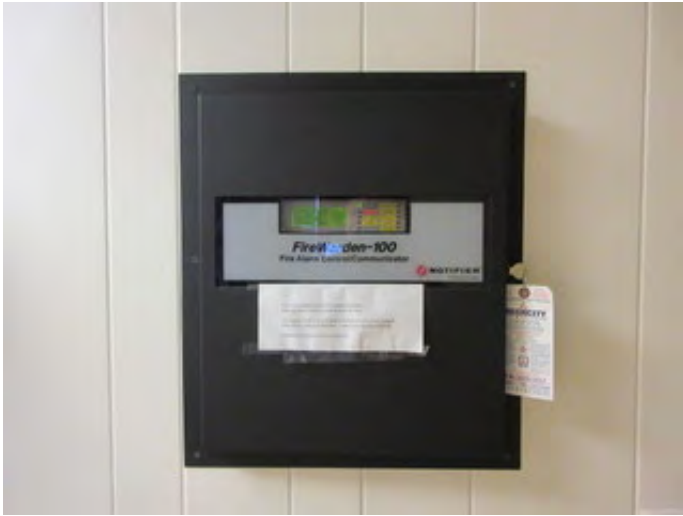
Fire Alarm Control Panel
