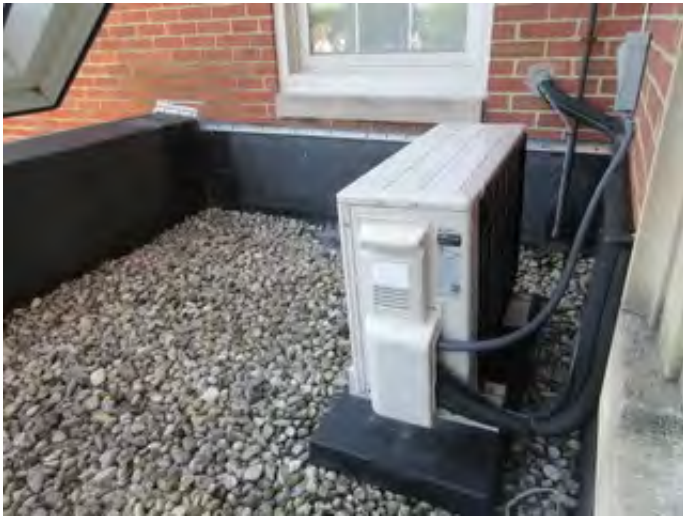
Ductless Split AC Condensing Unit
