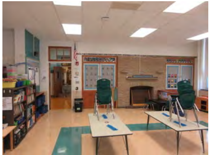
Classroom Fluorescent Light Fixtures
