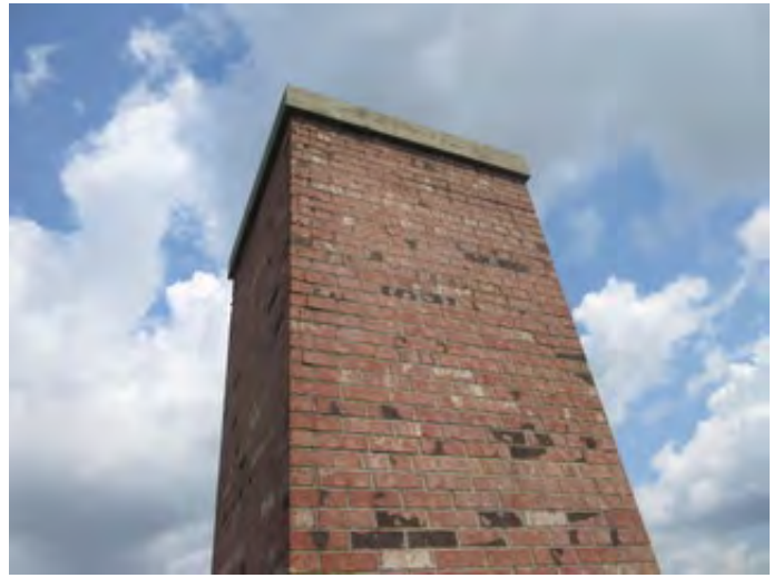
Chimney Tuckpointing Required
