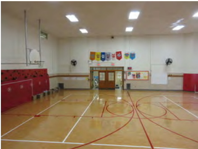
Gymnasium Fluorescent Light Fixtures
