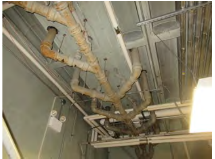
Sanitary Waste Piping
