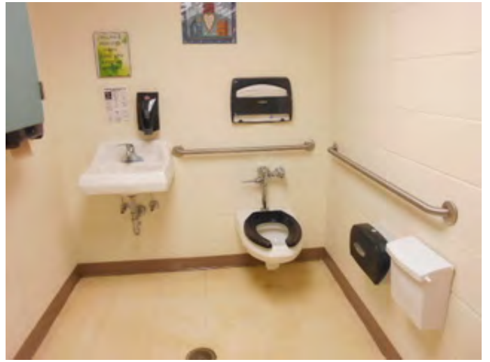
ADA Compliant Unisex Restroom
