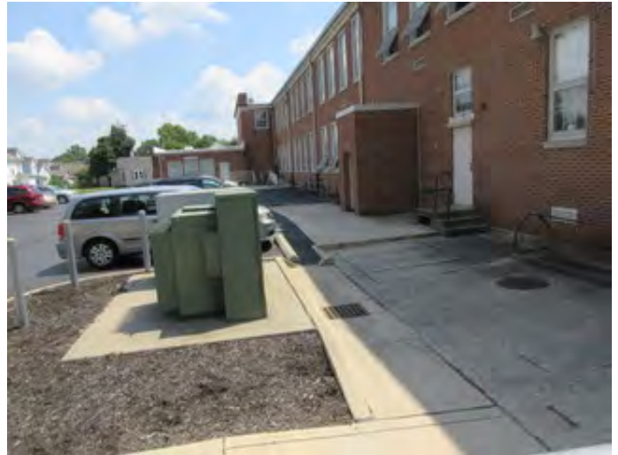
Pad Mounted Transformer
