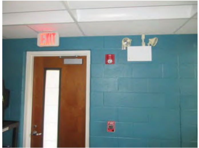
Exit Sign and Emergency Egress Lighting Fixture
