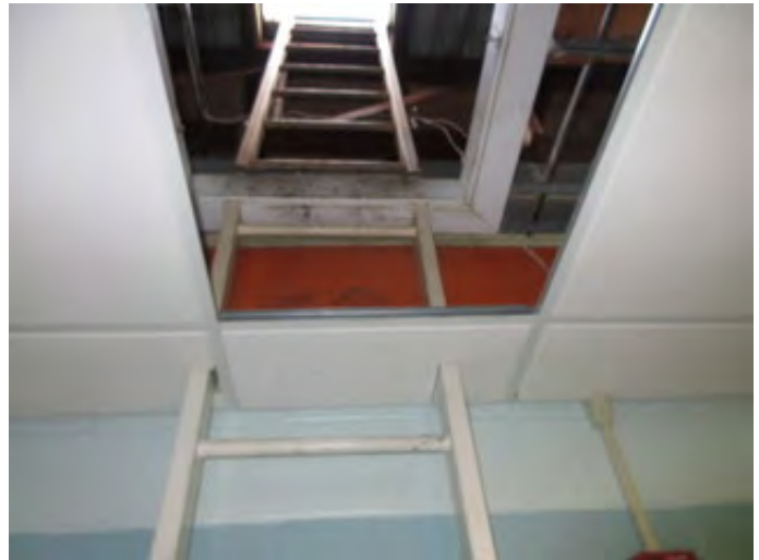
Unsafe Roof Access Ladder of the Original Construction
