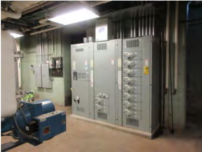
Main Electrical Distribution Panel
