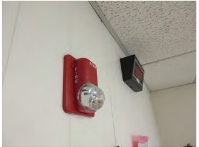
Fire Alarm Audible Horn and Visual Strobe Indicating Device
