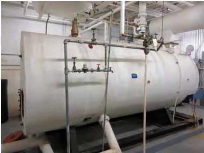
Natural Gas Fired Heated Water Boiler
