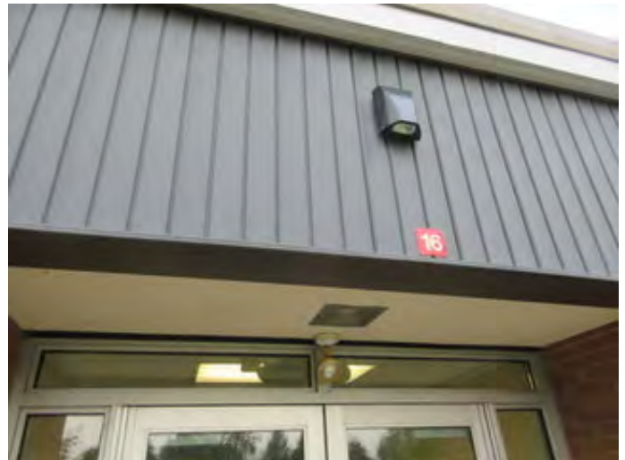
Entry Light Fixtures
