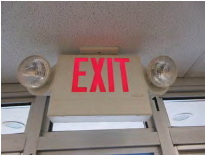
Exit Sign with Emergency Egress Lighting
