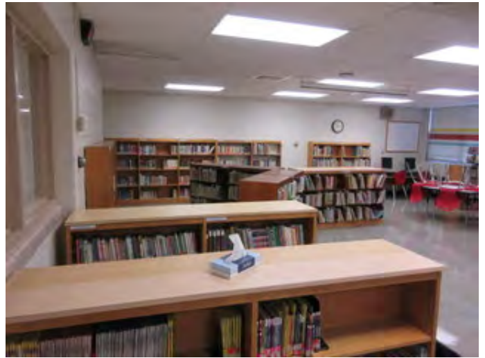
Media Center Fluorescent Light Fixtures
