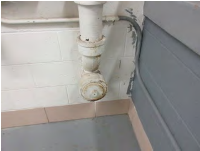
Sanitary Waste Piping
