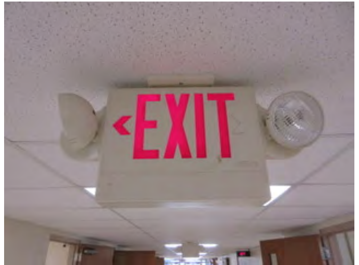
Exit Sign with Emergency Egress Lighting
