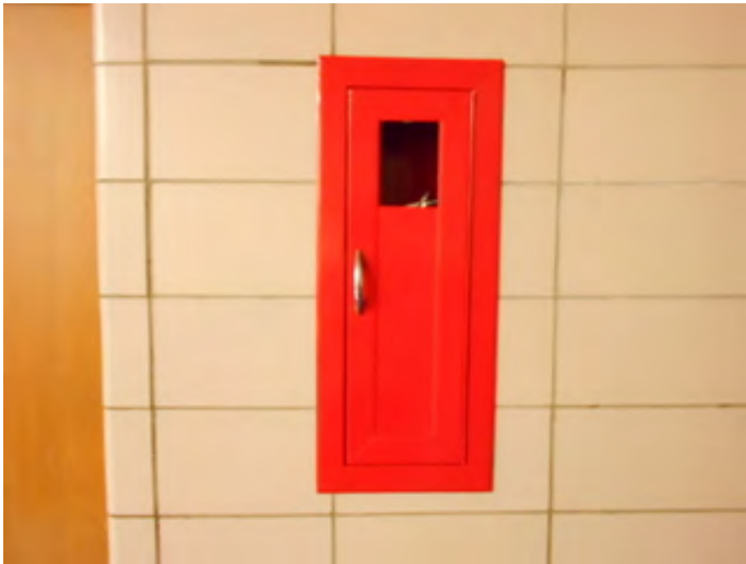
Compliant Fire Extinguisher
