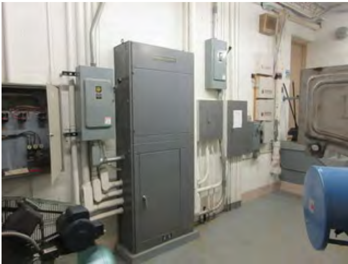
Main Electrical Distribution Panel
