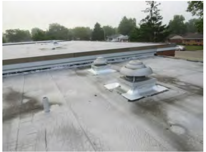
Waste Vent Piping
