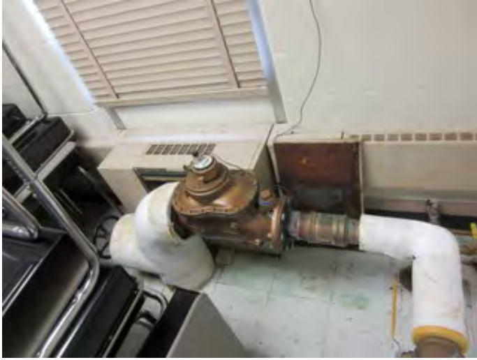
Incoming Domestic Water Service Line
