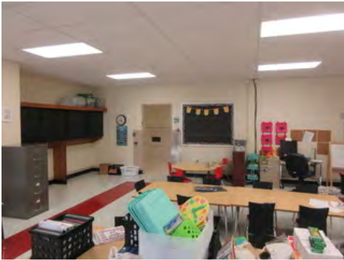
Classroom Fluorescent Light Fixtures
