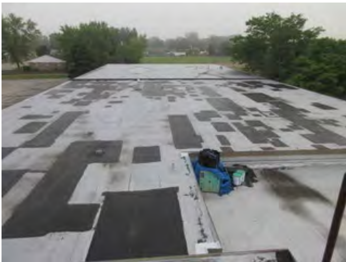
Excessive Patching and Stored Patching Materials
