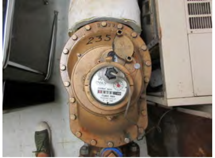
Incoming Domestic Water Service Meter
