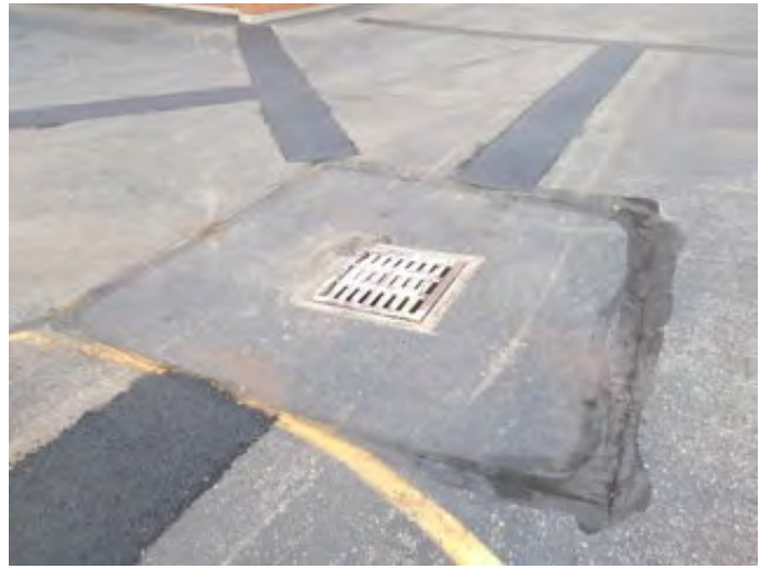
Play Area Asphalt and Catch Basin
