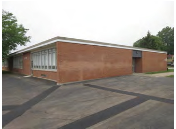
Exterior Masonry Cleaning Needed
