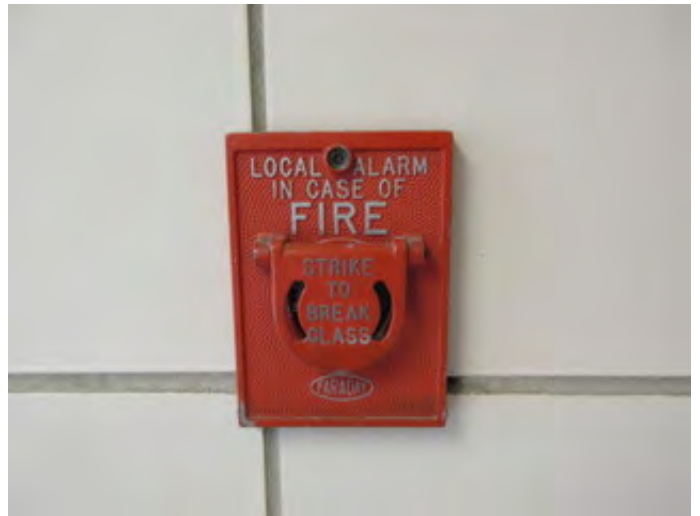
Fire Alarm System Manual Pull Station
