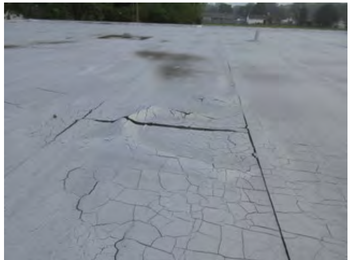
Typical Blisters and Cracking
