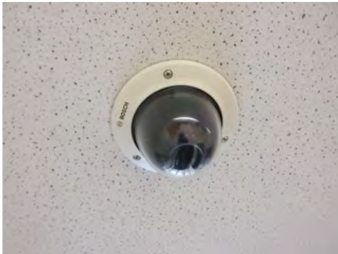
Security System CCTV Camera
