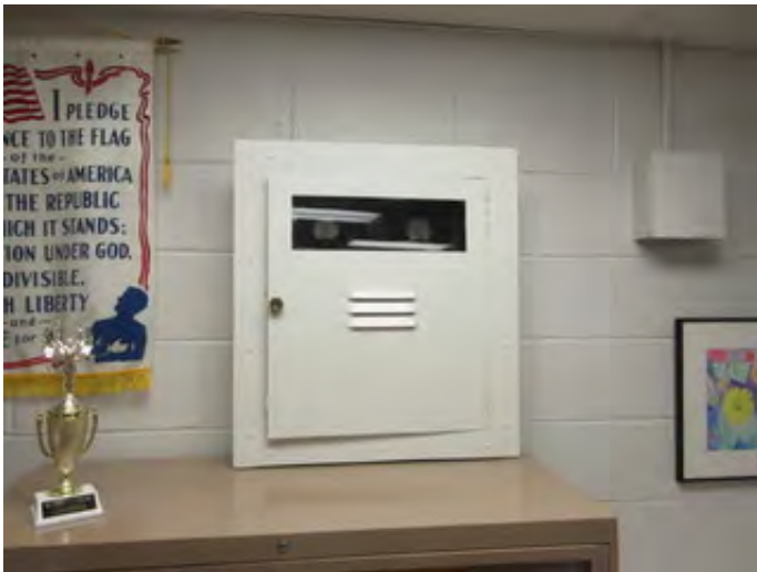
Fire Alarm System Control Panel
