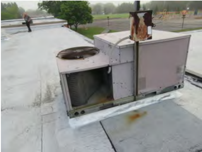
Roof Top Unit
