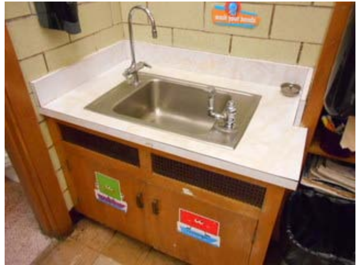
Classroom Sink With Deck Mounted Drinking Fountain
