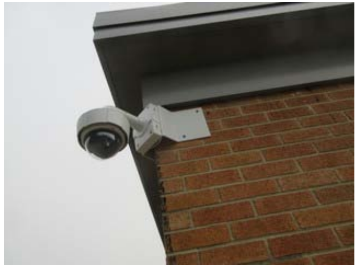
Security System CCTV Camera
