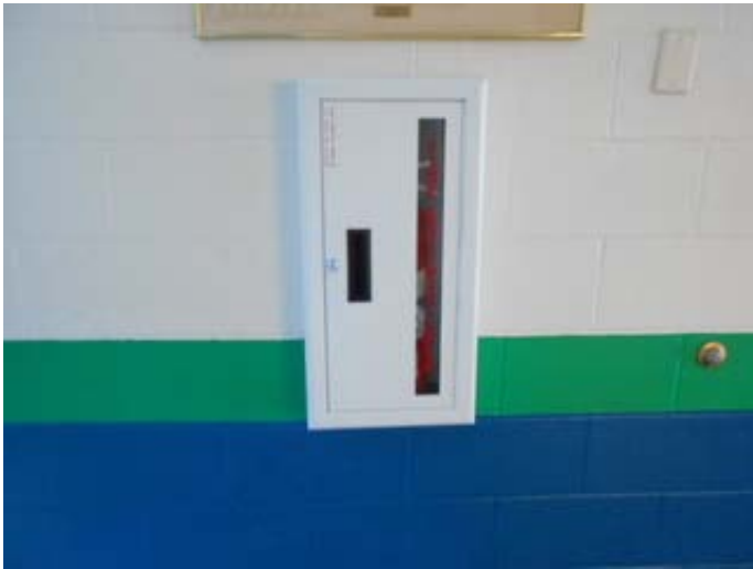
Compliant Fire Extinguisher
