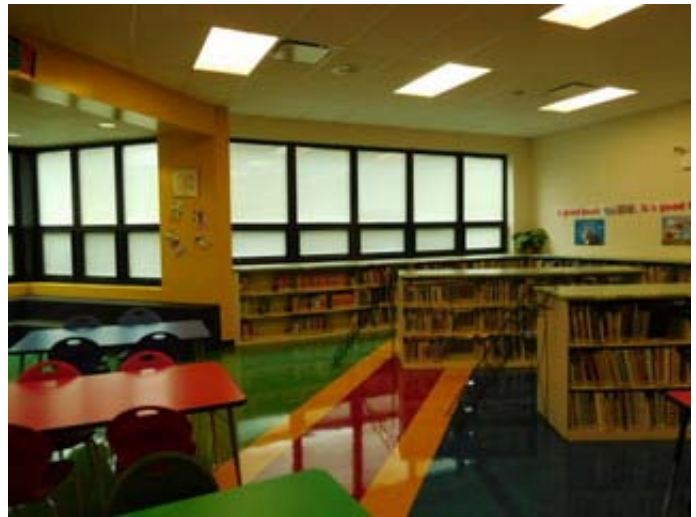
Media Center Fluorescent Light Fixtures
