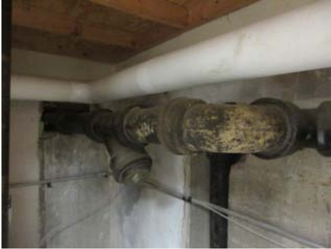
Sanitary Waste Piping
