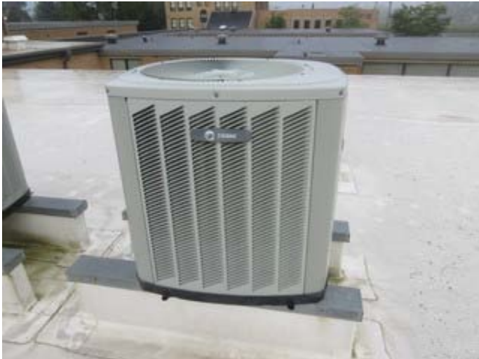
Roof Top Mounted Condensing Unit
