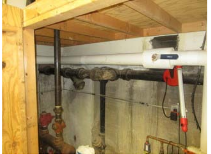
Sanitary Waste Piping
