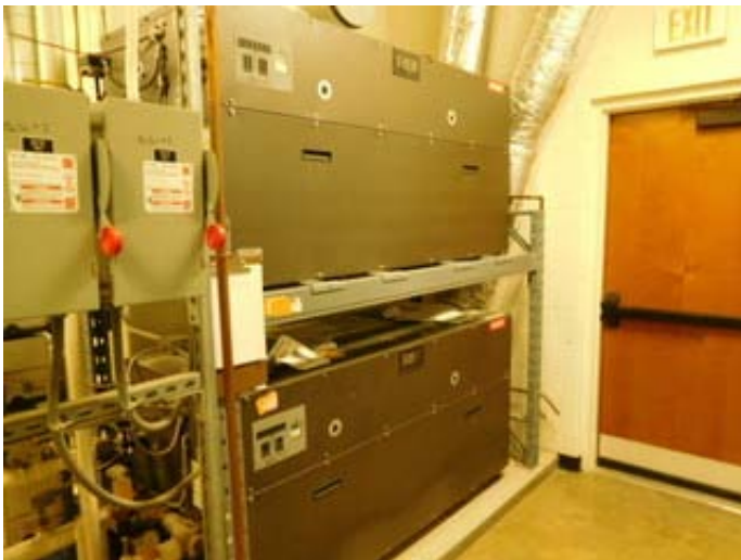
Natural Gas Fired Heated Water Boiler
