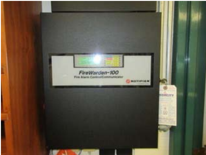
Fire Alarm System Control Panel
