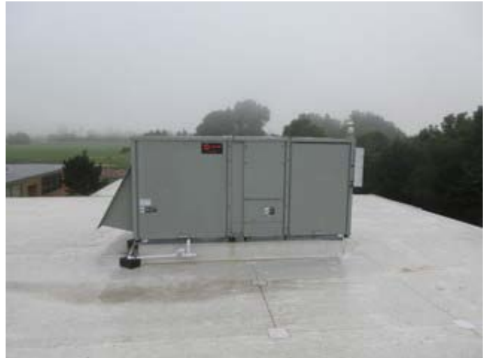
Roof Top HVAC Unit
