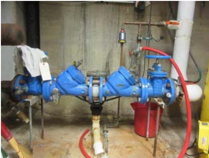
Incoming Domestic Water Service Line
