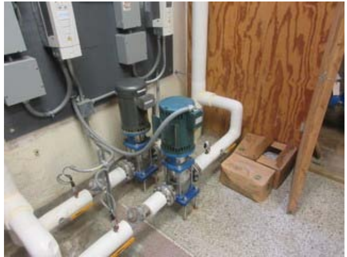
Incoming Domestic Water Service Booster Pumps
