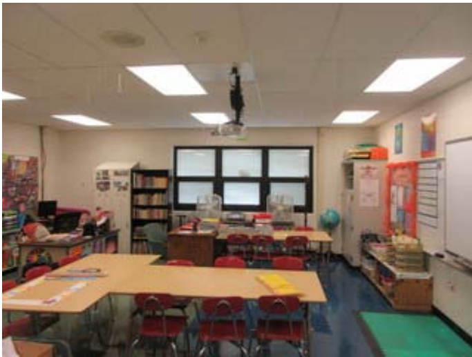
Classroom Fluorescent Light Fixtures
