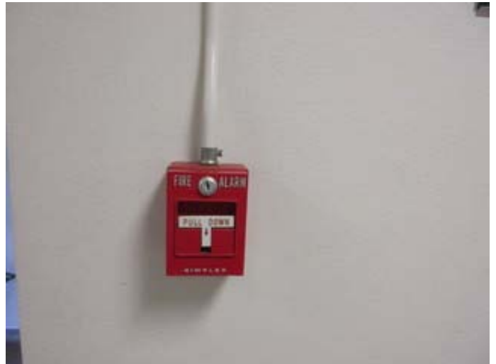
Fire Alarm System Manual Pull Station
