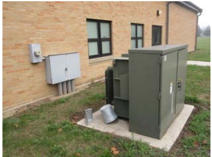
Pad Mounted Transformer
