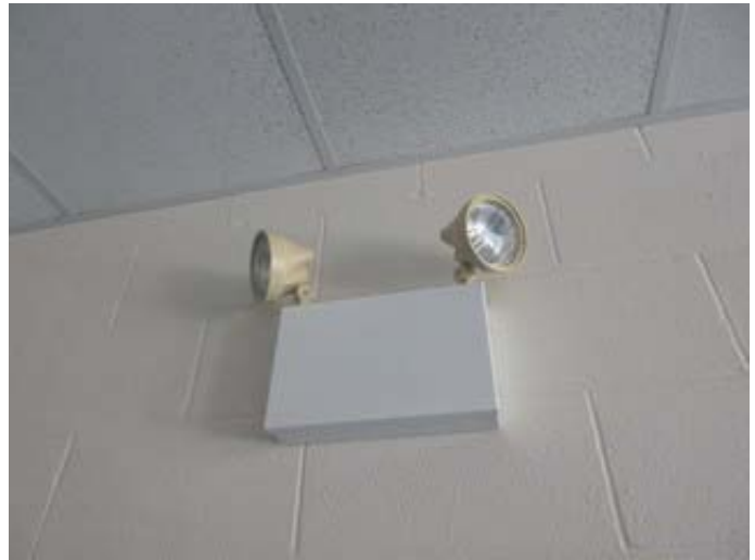
Emergency Egress Light Fixtures
